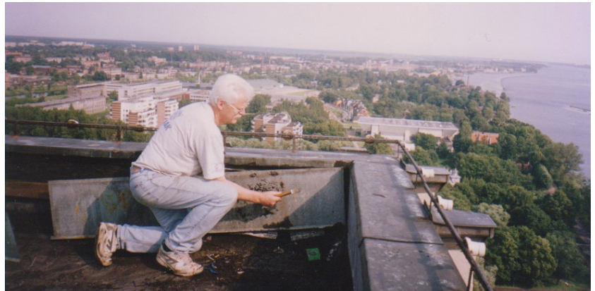
Figure 25. Tinsmith's work on the roof of the «Press House» (late 20th century).
